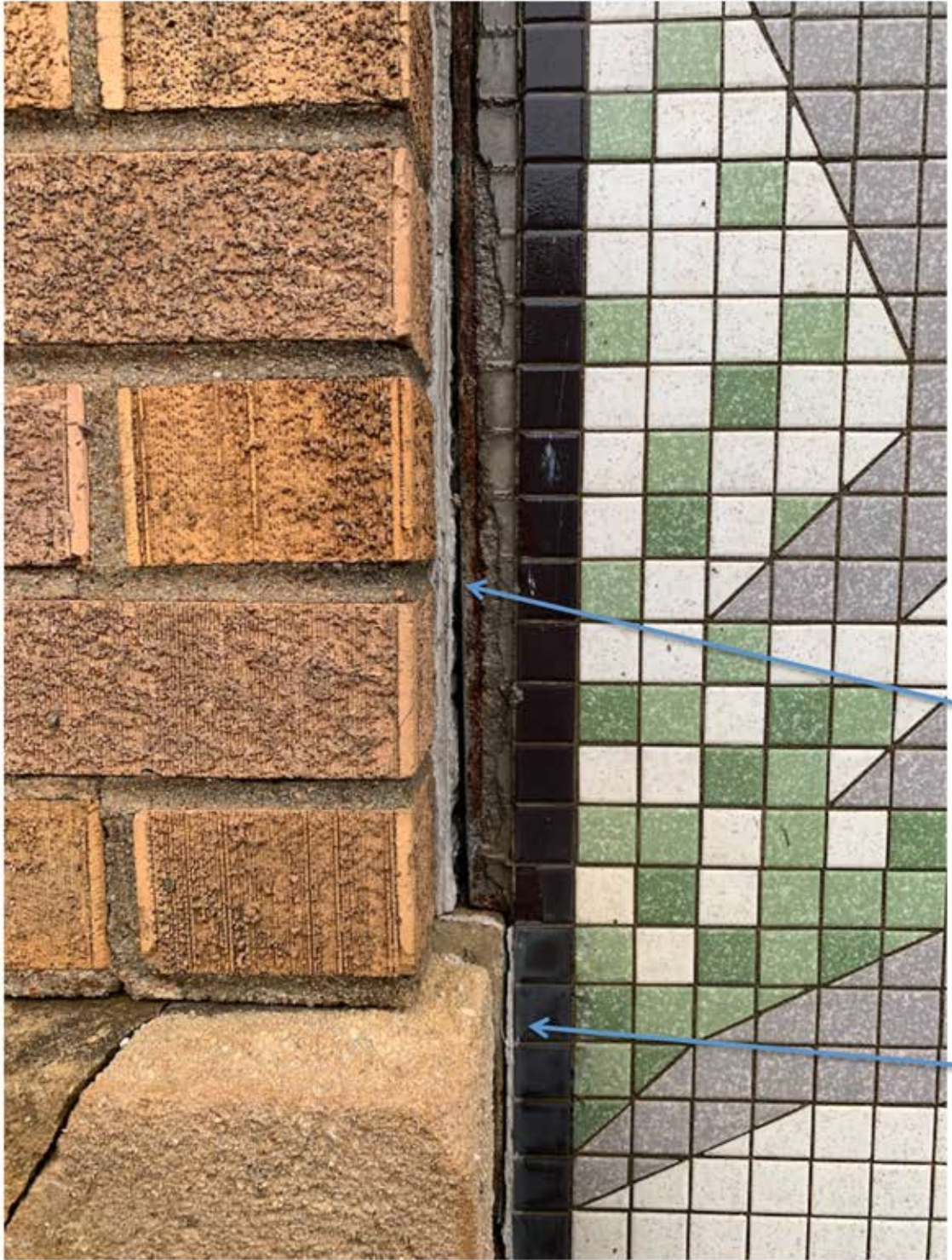
Seal of tile to brick wall is broken and not water tight, tiles are delaminating
